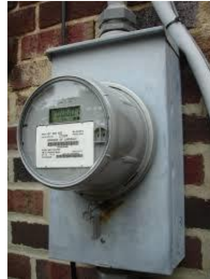
Your solar production meter. Runs forward only
